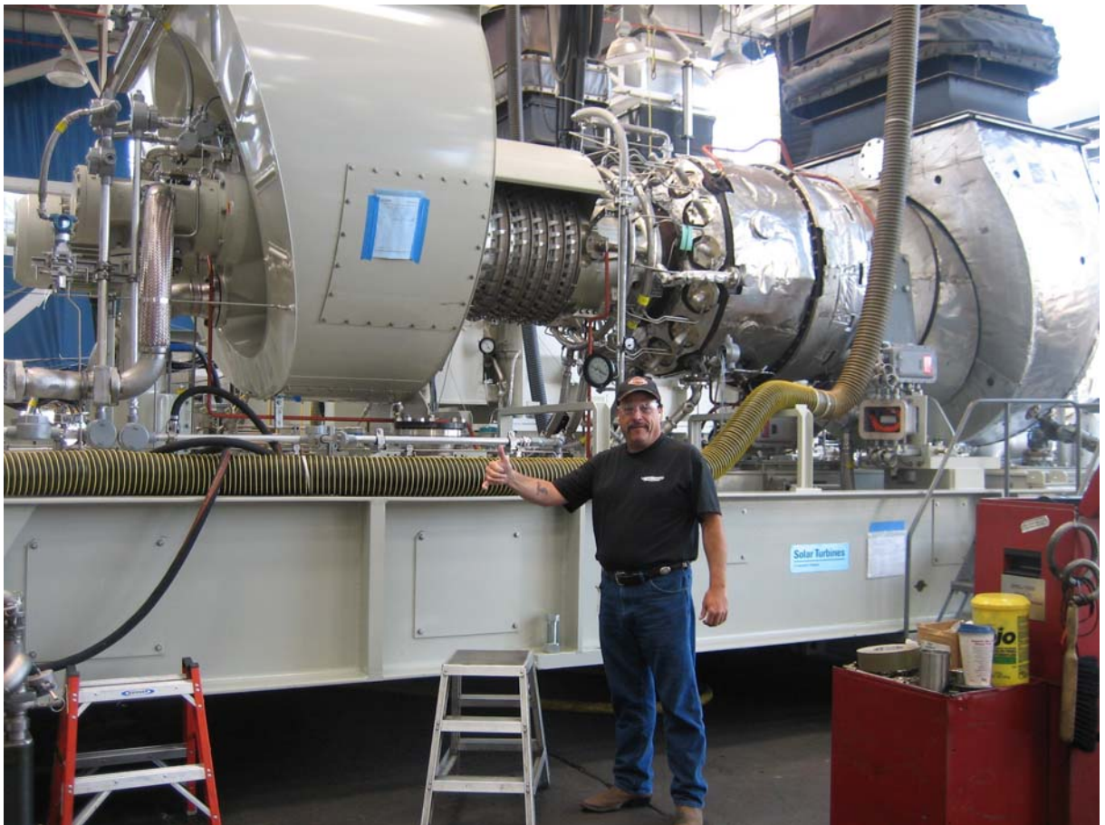
Solar Gas Turbine Compressor Package, Titan 130 rated 19,000 horsepower. Enagas Spain LNG
